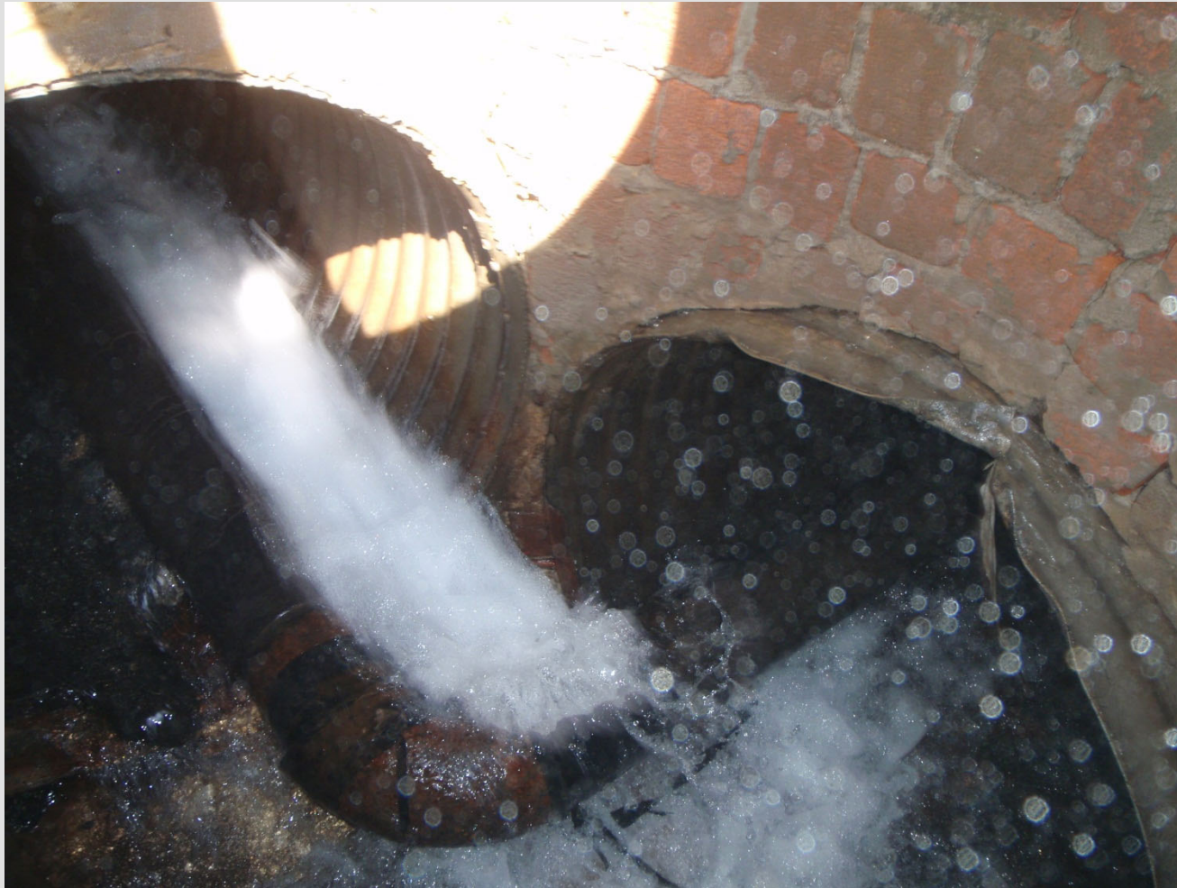
Thompson Spring non-contact reactor cooling water return flow
