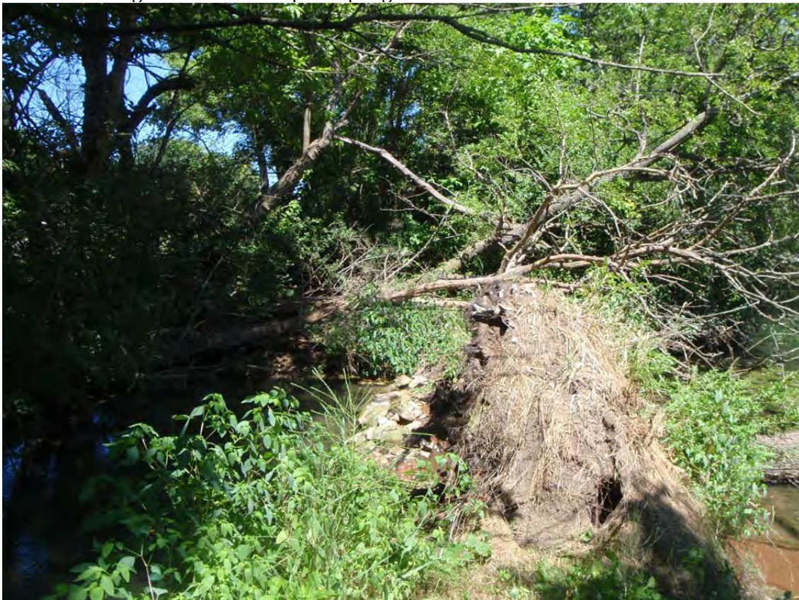
Figure 36. A large Trees Root Mass Breaching the Berm after Falling Over.
