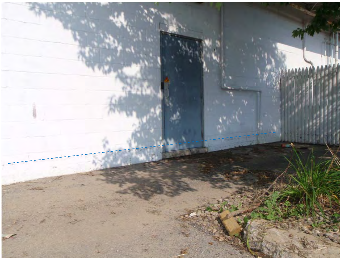
Figure 66. High Water Mark (11") from 8/12/2009 Event on the West Side of the Your Building Center Building
