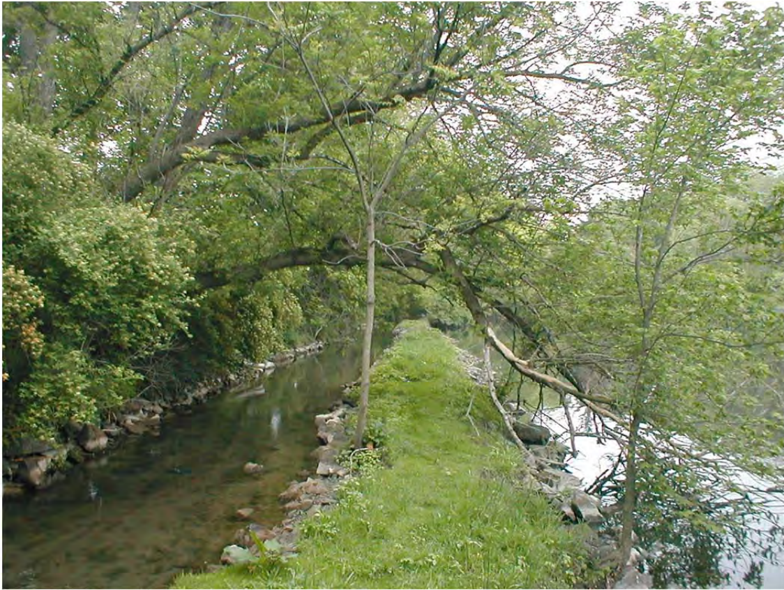
Figure 35. The Thompson Spring Diversion Berm in an Ideal Section
